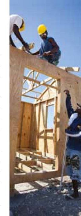
☞ At the La Piste camp in Port-au-Prince, the IFRC supported a team of builders, all of whom are deaf, to construct shelters in 2010.
